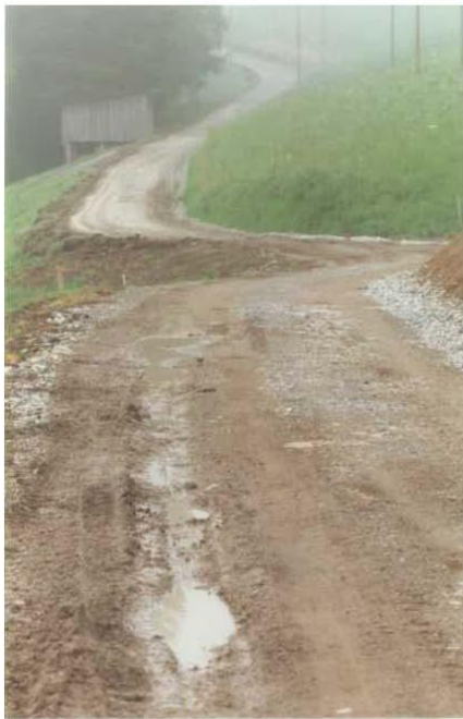
Poor or muddy road conditions before repair
