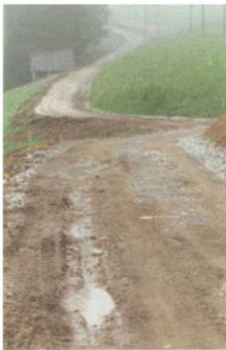
Poor road conditions before TerraDry treatment
