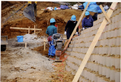
Native soil was used for infill, eliminating the time and expense of importing soil.
