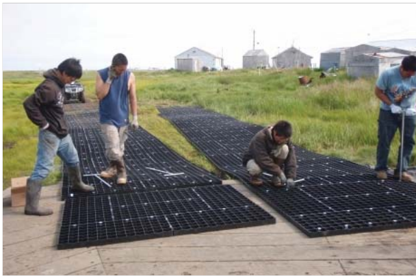
The trailbuilding units formed an interconnected structural mat pavement system. Photo courtesy of the author.
